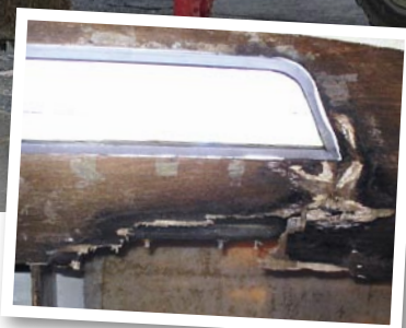
Leaking windows meant a lot of interior joinery was rotten
