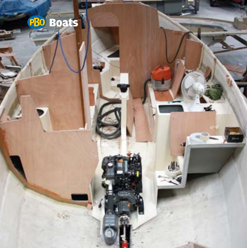
The engine and stern gear have been fitted, as have the bulkheads, which are bonded and laminated to the hull
