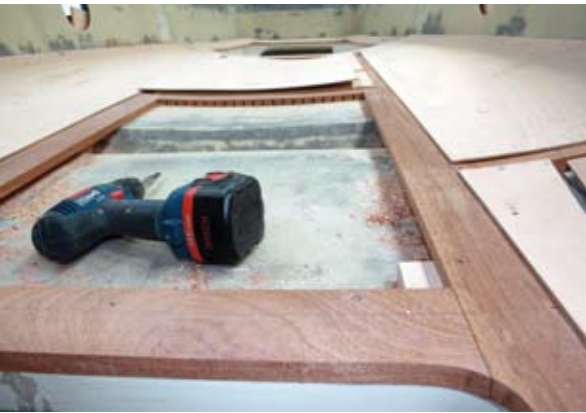
Hardwood is used for the framework, grooved on the reverse face to allow it to bend to fit the deckhead
