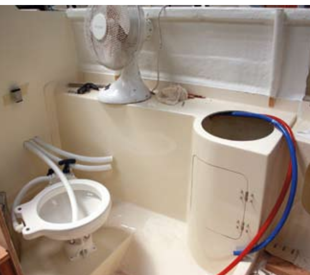
Pipes for the heads and for the hot and cold water to the sink are fed through the bulkhead and interior moulding. The inside of the hull has been partially flow-coated (painted with thinned gel coat) to give a smooth finish
