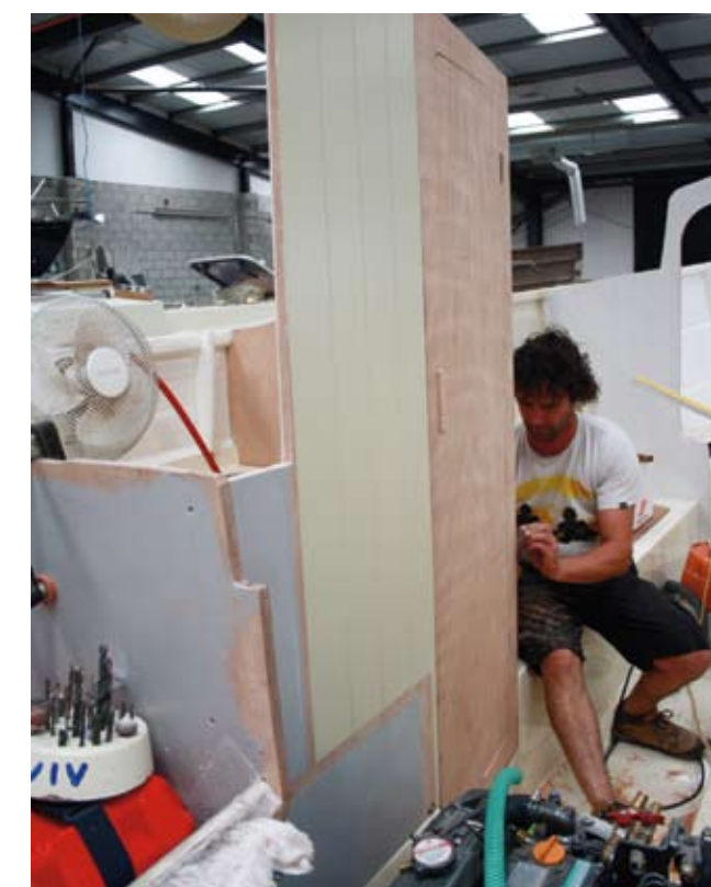
The last of the major interior dividers, the heads bulkheads and door, are fitted. The door opens forward
