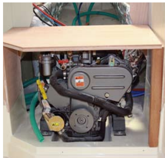
Day-to-day engine access will be from the forward end. Here the casing is built in timber, but it will be partially replaced by a moulding on future boats
