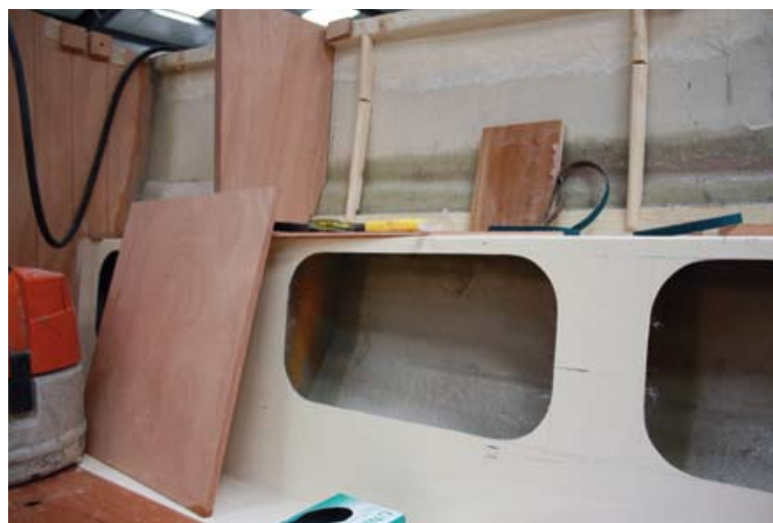
Although the interior moulding forms most of the structure, a fair amount of joinery is still needed. Here the vertical supports for the cedar battening have gone in above the moulding and the timber for the hullside locker units is being fitted
